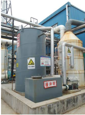
喷淋塔区围堰
